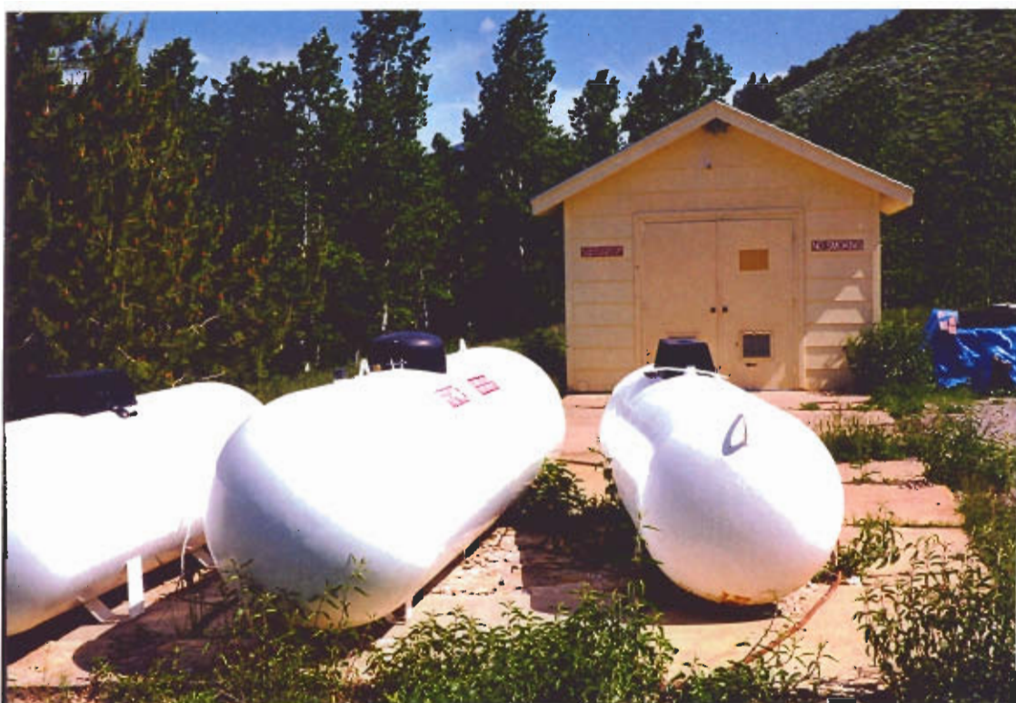
6 – View looking northeast at three propane tanks and electric generator building in the background.
