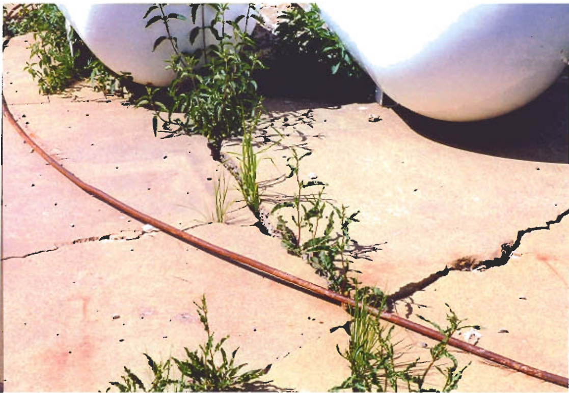
8 – View looking southwest at propane tanks and concrete pad, which is deteriorating.
